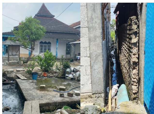
FIGURE 2. Open Sewerage at Ibn Cholil Islamic Boarding School
